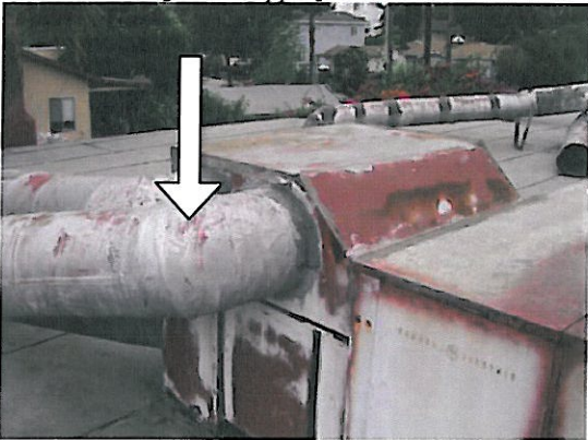
3. Peeling lead-containing silver paint (also ACM) on the roof-mounted HVAC unit housing and ductwork of the Factory [Bulk Sample I.D. Pb-09-SLVR, containing 900 ppm].
