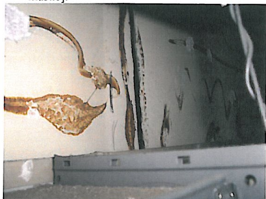
18. ACM brown wall mastic (including concealed material) observed in a Storage Room, Sewing Room and Men’s Restroom, totaling about 25 ft 2 observed [Sample I.D. MASTIC-27-01, -02, -03, containing 1-2% CH].
