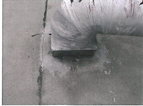
8. ACM silver/gray mastic associated with roof penetrations, totaling about 100 ft 2 [Sample I.D. RFMAS-06-01, -02, -03, containing 3% CH].
