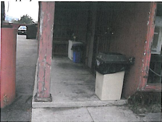
5. Chipped and peeling lead-based brown paint on an exterior wood support column and wood utility housing of the Factory [Bulk Sample I.D. Pb-14-BR, containing 38,000 ppm].
