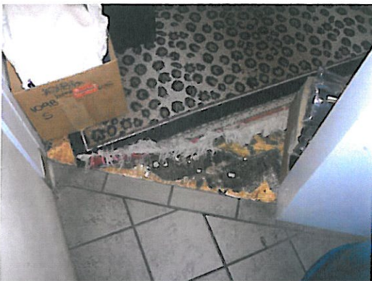
17. ACM black mastic present below non-ACM leveling compound in the Office Storage Room, totaling about 10 ft 2 [Sample I.D. MISC-24-01, -02, -03, containing 3% CH in the mastic, only].
