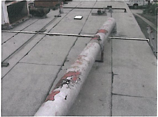
12. ACM and lead-containing silver texture coating on “round” HVAC ductwork, totaling about 400 ft 2 [Sample I.D. MISC-11-01, -02, -03, containing 3% CH].
