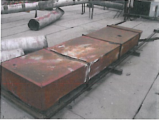
1. Intact lead-based red paint on metal HVAC equipment housing and ductwork on the Roof of the Factory [Bulk Sample I.D. Pb-08-RD, containing 21,000 ppm].
