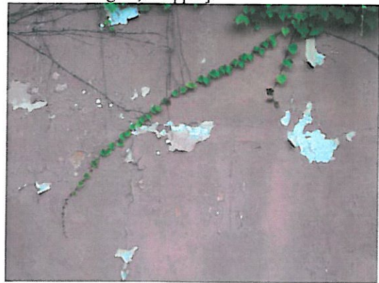
4. Chipped and peeling lead-containing red paint on the exterior stucco walls of the Factory [Bulk Sample I.D. Pb-10-RD, containing 900 ppm].
