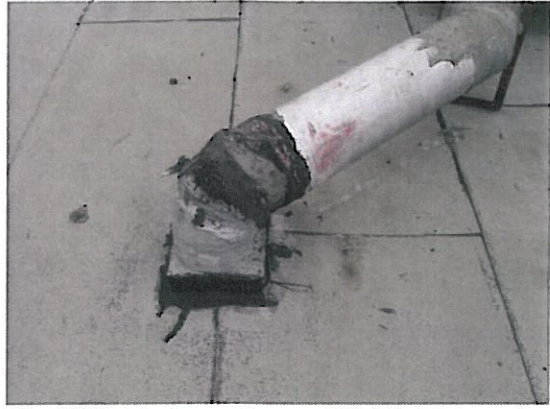
10. ACM black mastic on HVAC joints and seams, totaling about 20 ft 2 [Sample I.D. HMAS-09-01, -02, -03, containing 2% CH].
