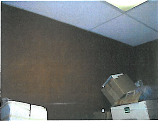
19. ACM concealed wall mastic (assumed present behind wood and cork wall panels), totaling about 500 ft 2 [I.D. MASTIC-AAA, assumed asbestos containing by SCA].
