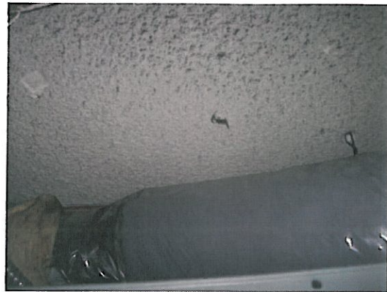
14. ACM sprayed-on acoustical ceiling finish, totaling about 1,000 ft 2 (occurring above non-ACM laid-in ceiling tiles) [Sample I.D. CLTX-17-01, -02, -03, containing 5% CH].
