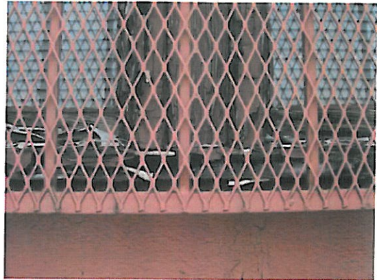
2. Severely chipped and peeling lead-based red paint on the exterior wood window frames of the Factory [Bulk Sample I.D. Pb-11-RD, containing 67,000 ppm].
