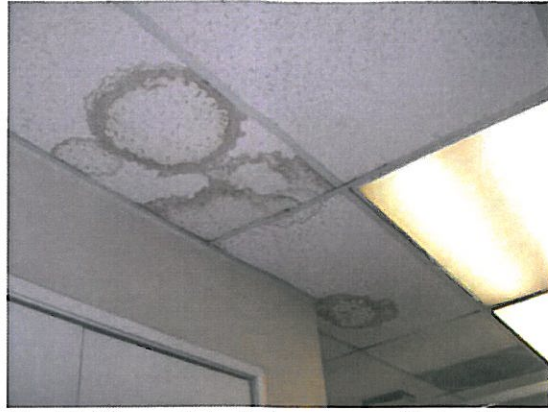
20. Visible water stains on ceiling tiles, attributed to roof leaks.
