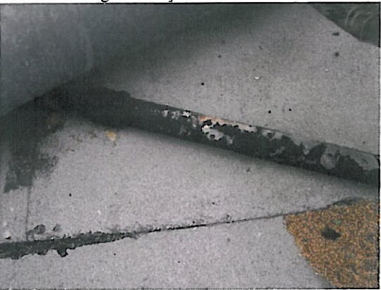
11. ACM black, tarry wrap/coating on 1” and 2” pipes on the roof, totaling about 30 ft 2 [Sample I.D. MISC-10-01, -02, -03, containing 3% CH].
