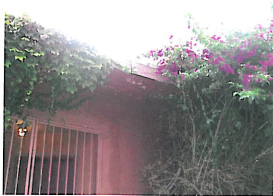
6. Severely chipped and peeling lead-based red paint on the exterior wood fascia of the Factory [Bulk Sample I.D. Pb-19-RD, containing 22,000 ppm].
